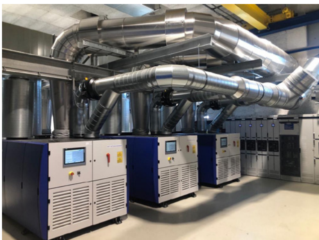
The new HST compressors will save around EUR 175'000 per year
