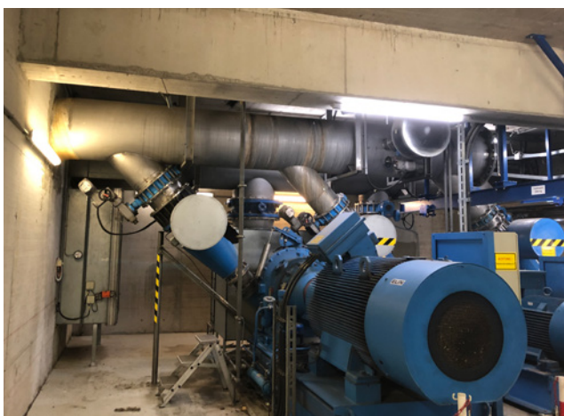
The legacy compressors were located underground to reduce noise pollution
